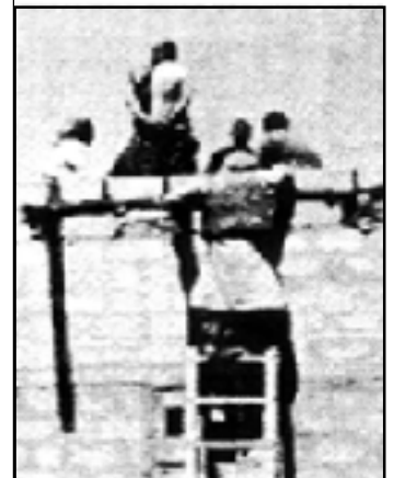
Training of builders in hazard-resistant construction techniques is best carried out through practical exercises and advice on-site.
